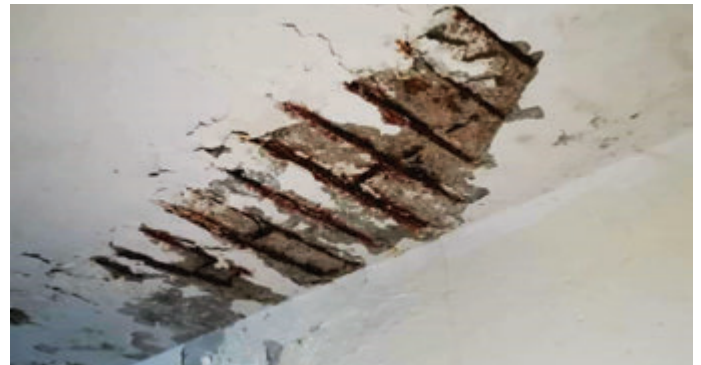
Figure 2: Dampness from water leakage caused spalling of concrete soffit
