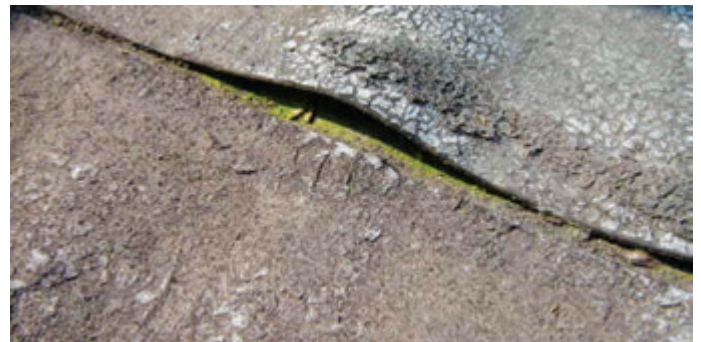
Figure 21: Premature failure of modified bitumen membranes
