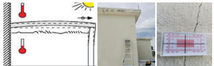
Figure 18: Crack expanded by 0.5mm at noon
